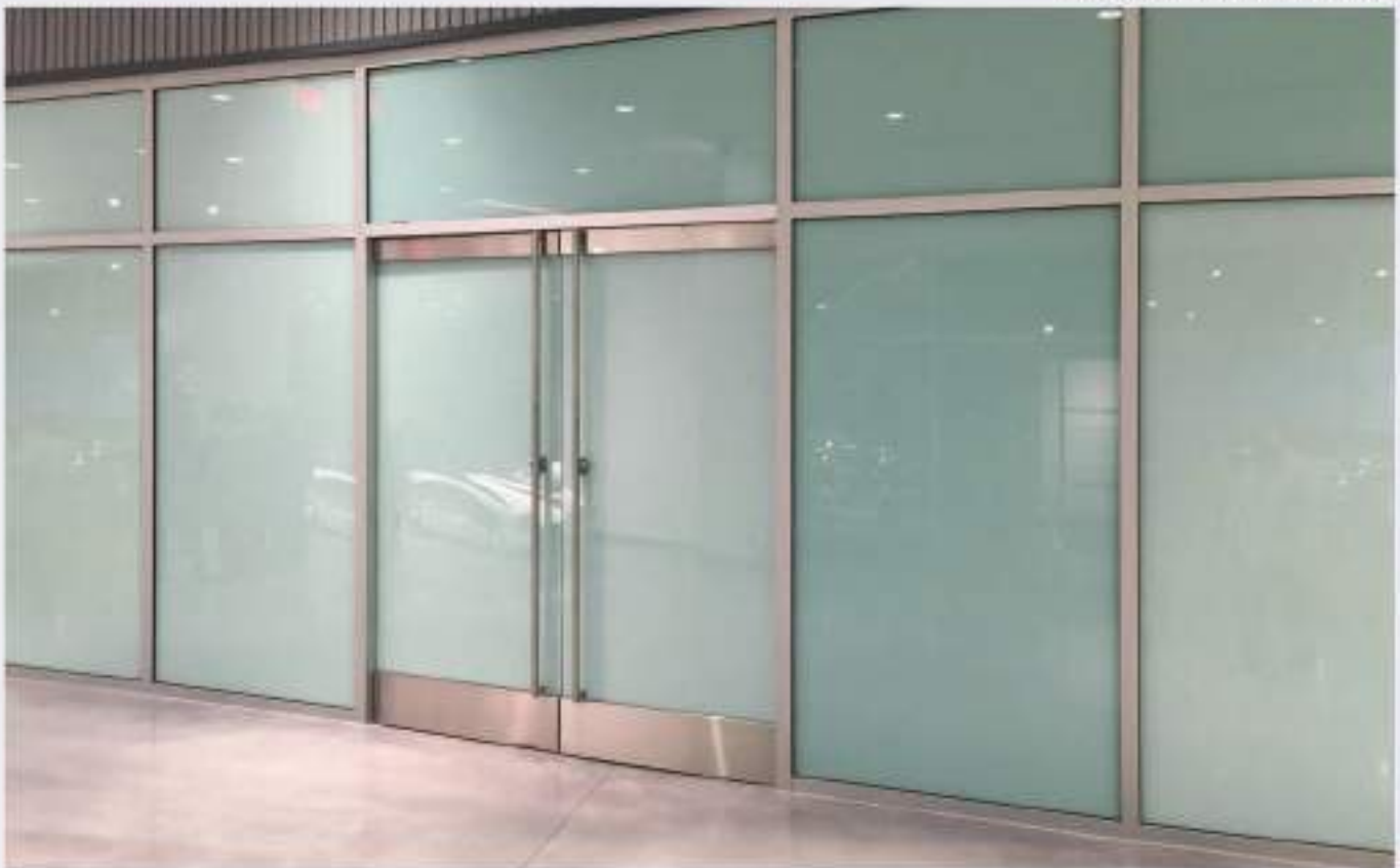
Entrance System & Storefront with Aquamarine Laminated Glass
